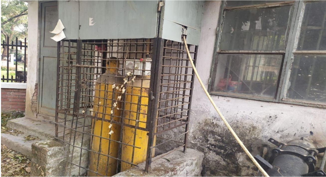
Figure 6. 11 Nazrul Islam Hall Pump Station
