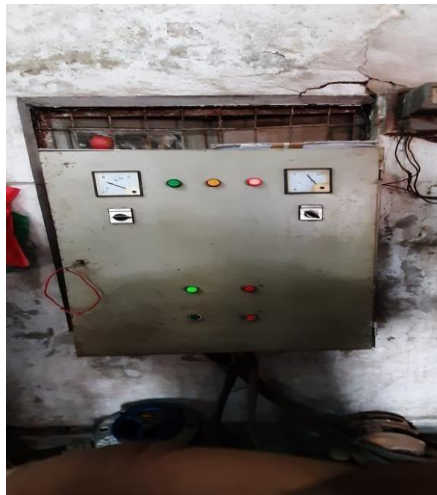
Figure 6. 8 Ampere and voltage meter
