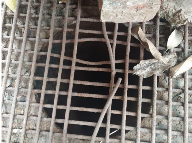
Figure 6. 2 Housing pump (pumping station near DSW office)
